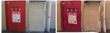
(c) Fire Hydrant
